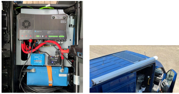
(a) Power management system with Li-ion battery, solar charger, and inverter (below) (b) Solar panel on the roof of the van
